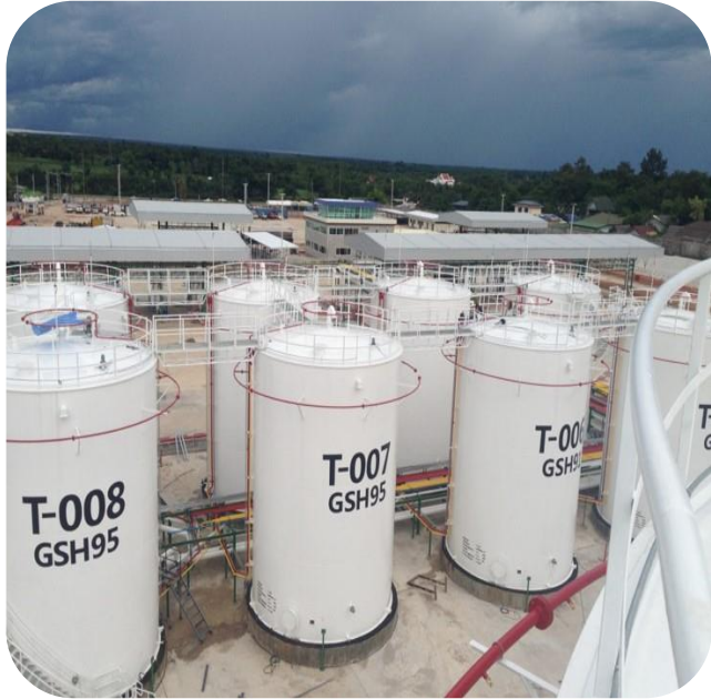
Storage Tanks with Cooling Rings
