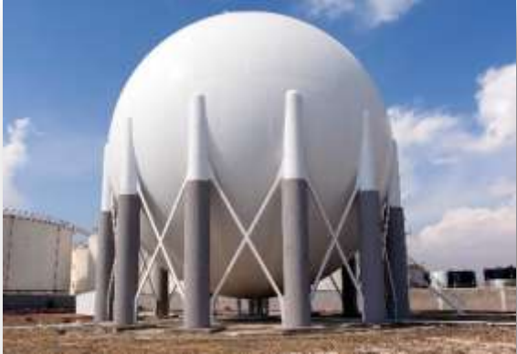
LPG Tank and System
